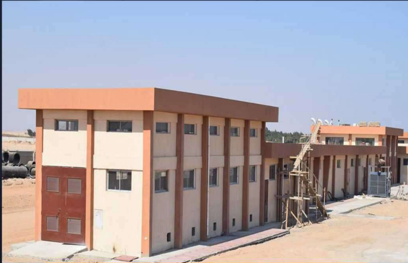
WATER LIFTING STATION 15MAY CITY (5MVA) (Residential Project)
